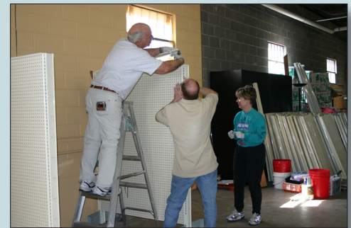
Zonta Club of Denver II members renovating the Baby Bucks Store, where students get rewards for good attendance and grades
